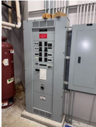
Main Distribution Panel 'MDP'
