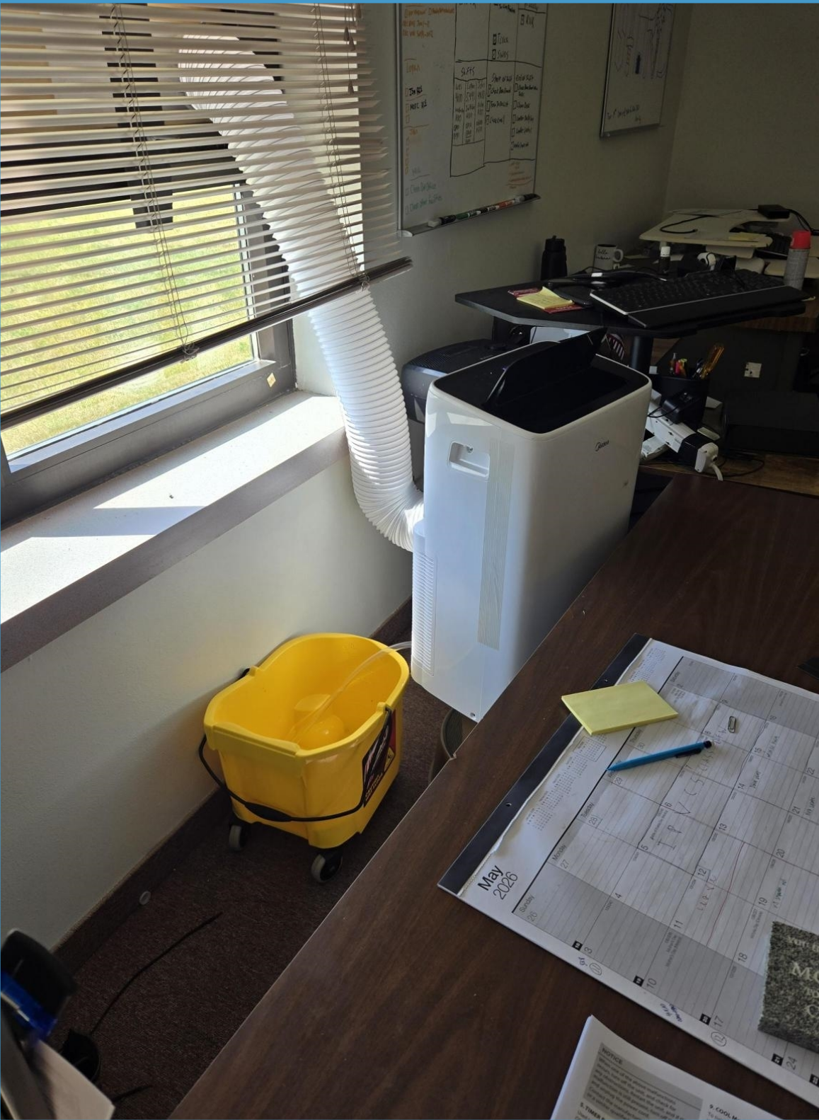
Temporary fix to HVAC in FAA Tech Ops space
