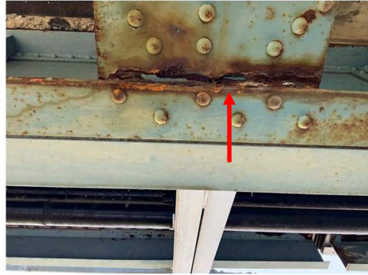
Gusset Plate Section Loss
