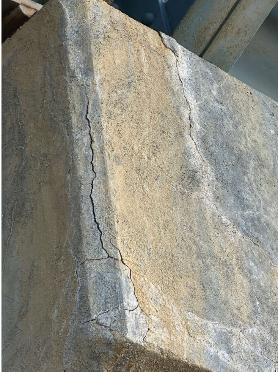
Cracks in west column cap
