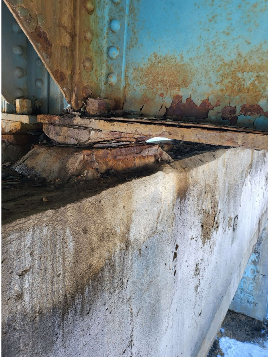
Typical bearing with some concrete spalls and pack rust
