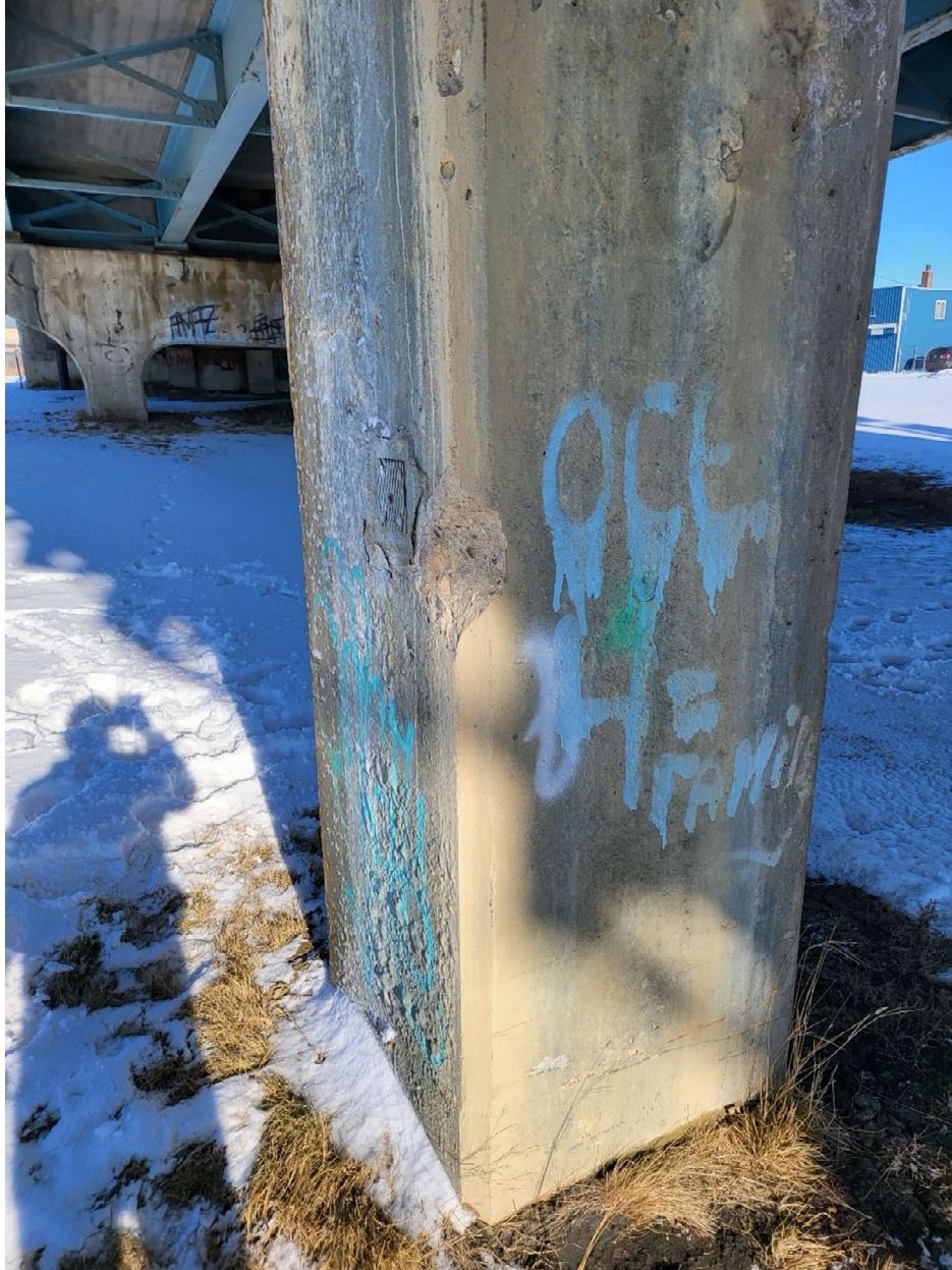
Spall in southwest corner of west column
