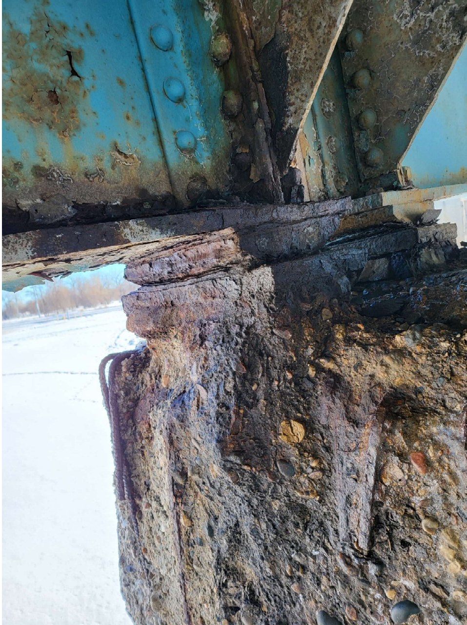
Pier 3 Span 2 East Girder Bearing. Eroded grout pad shown under northeast corner of the bearing.
